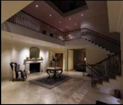
A state-of-the-art residential lighting control system
