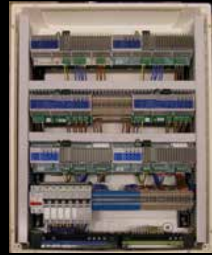
A bespoke DIN rail modules enclosure allows for easy installation of HomeWorks QS and gives a clean and stylish finish
